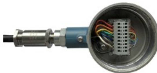
Fig.4.9 Nine-core shielded cable connection
